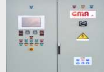
Control Panel with HMI
